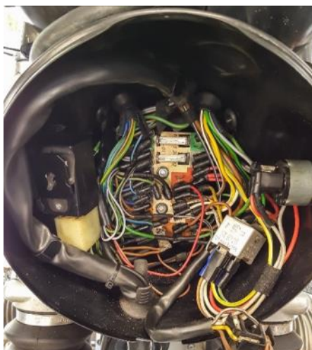
Now that is how the inside of the headlight should look...
